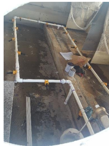
Return piping with directional jets installation, adjusted to prevent stagnant areas and particle build up in basin.
