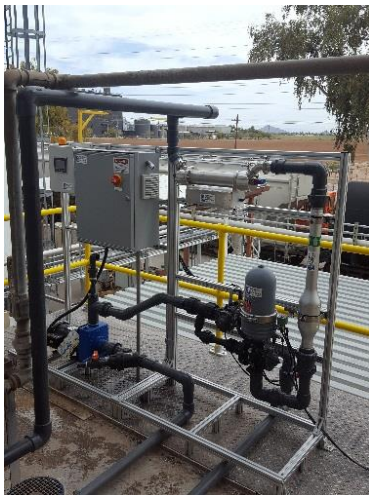
The conditioning system installed at the condenser continuously cleans and treats the basin water to maintain best performance.
